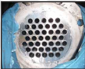
Gascooler gas pipings
